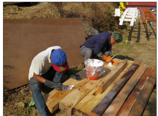
Application of protective coats: first coat with a primer (in white), second coat with an oil based paint (in brown). ©Vincent Pena, Rapcha, Solokhumbo district, Nepal
